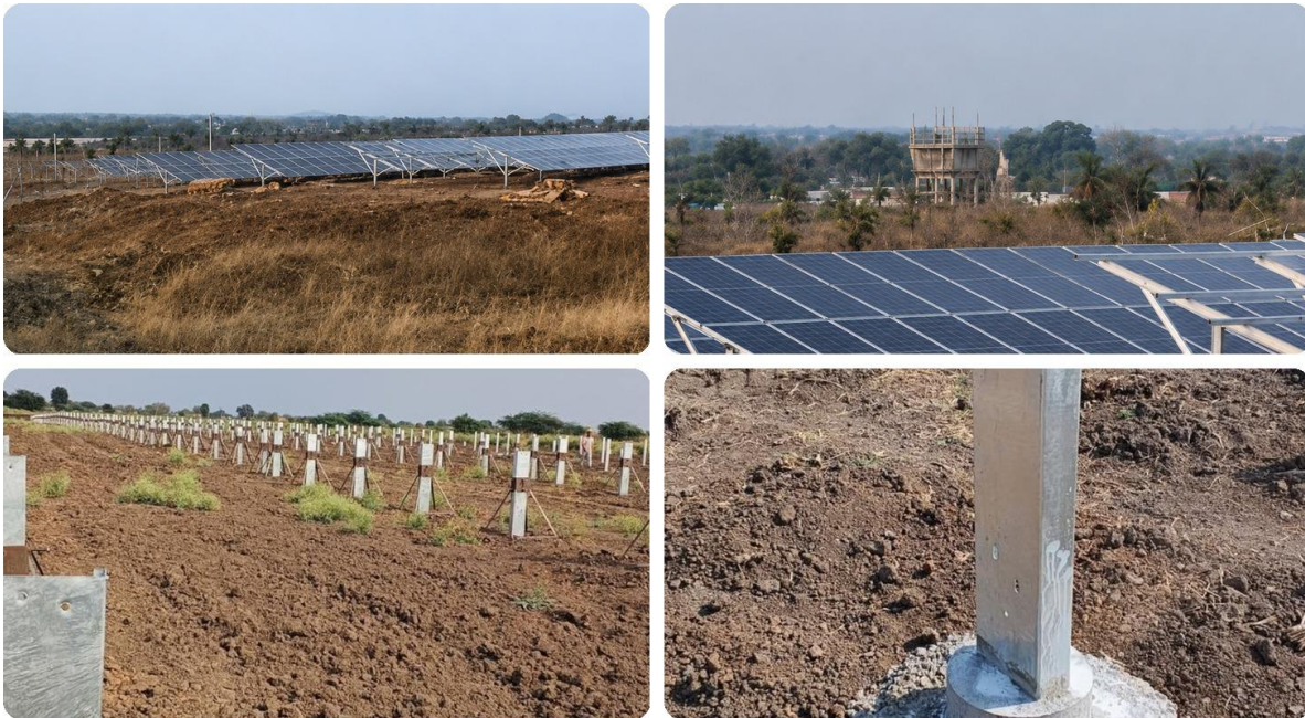
Figure 2. Clubbed construction views for the 3.24 MWp Ujjain project: installed array, modules, access road and foundations.
